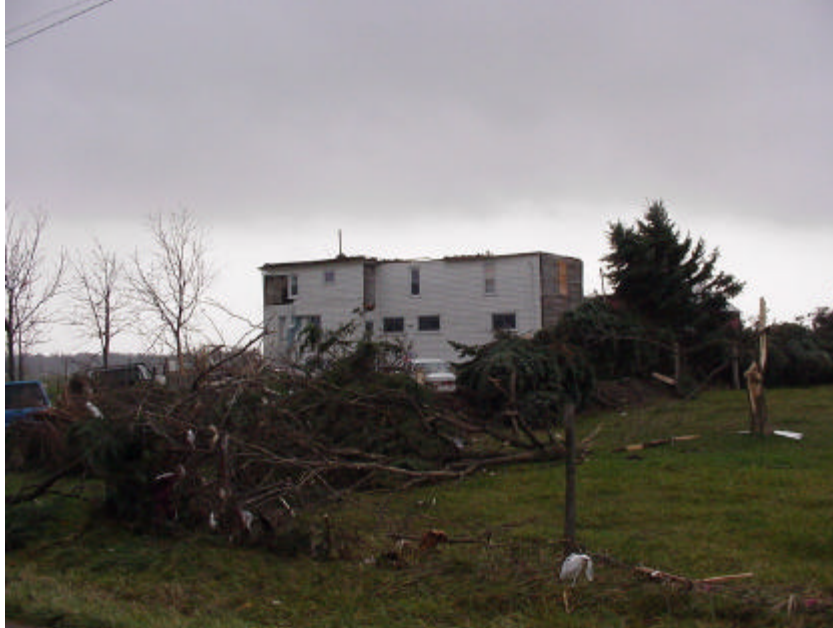
Tornado damage along Ashland County Road 620 just west of Albion.
