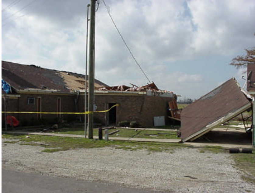
A church and parsonage near the town of Heafer were badly damaged by a tornado on November 9th.
