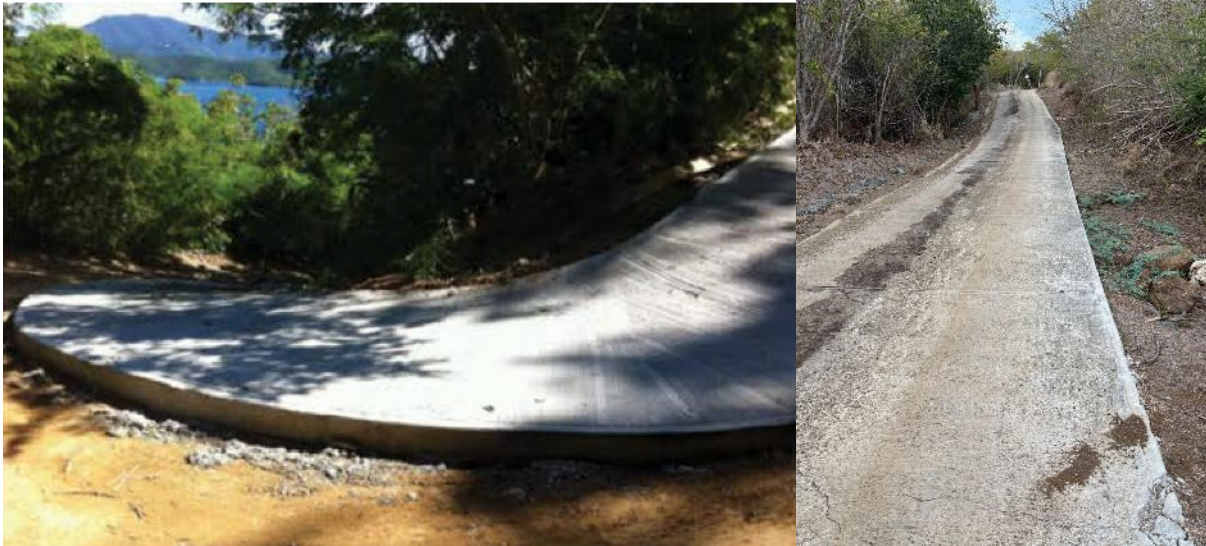
Figure 3: Examples of stabilized paved roads and best management practices ( Kitchell et al., 2021 ).
