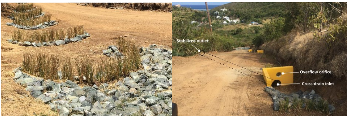
Figure 2: Examples of stabilized dirt roads and best management practices ( Kitchell et al., 2021 ).
