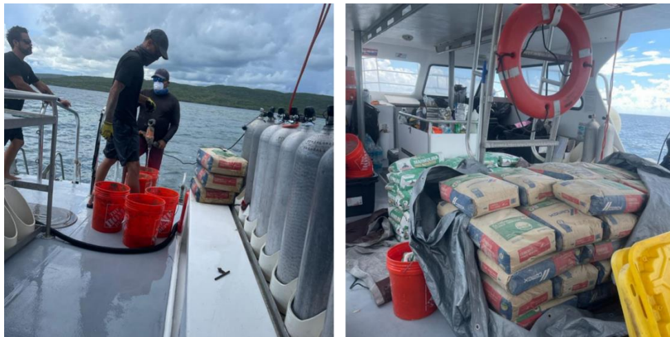
Figure 2. Cement cargo and mixing process aboard to Sea Ventures Marine Response Unit vessel.
