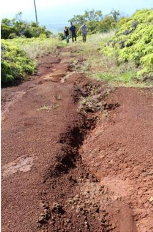
FIGURE 4 EVIDENCE OF GULLYING IN FORMER AGRICULTURAL ROADS, WEST MAUI, HAWAII.
