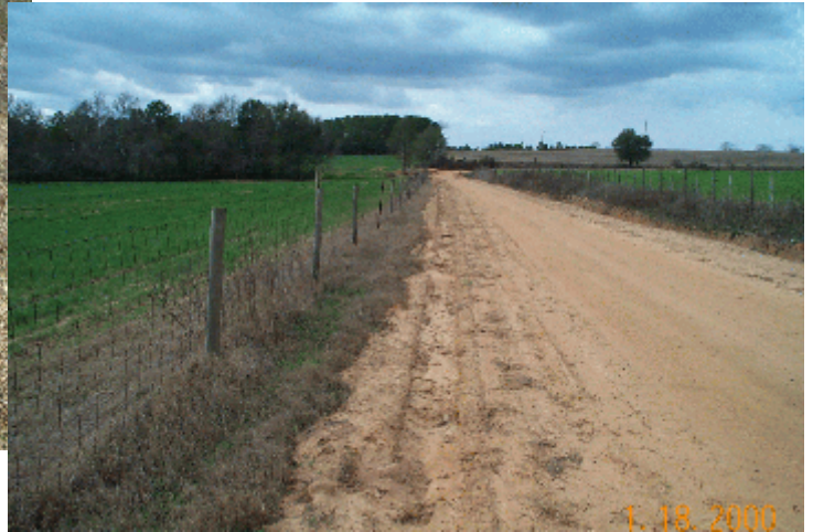
False ditch created by shoulder traffic and rutting
