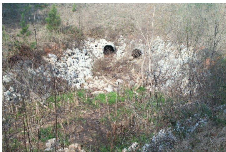
Mechanical Riprap Basin Revetments Vegetated Naturally with Willows (Growth Age is a Beaver-Pruned Four Years)
