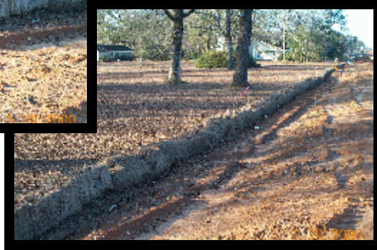
Ineffective Placement (Parallel to Flow)
