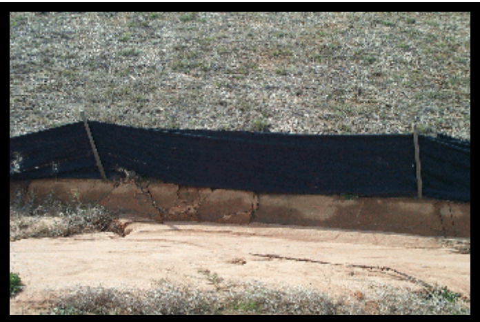
Exhibit 6.2b - Improperly placed and erected silt fence.
