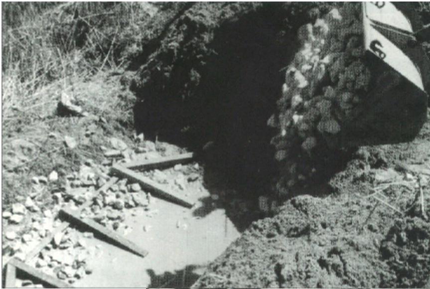
Preparing Foundation of Structure. Rock Fill (Optional) Placed in the Foundation of Structure to the Level of Inundation. Soil Fill May be Used When Inundation or Perennial Flow Will Not be Encountered.
