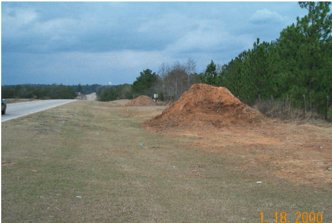
Soil stockpiles located on a well vegetated hillcrest and away from concentrated flow channels
