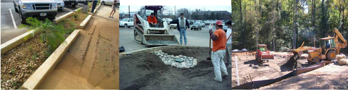
Figure S2.7. Construction sediment can easily damage bioretention filter bed (left). Block inlets during construction (middle) and/or install temporary silt fence around perimeter of bioretention during construction (right).
