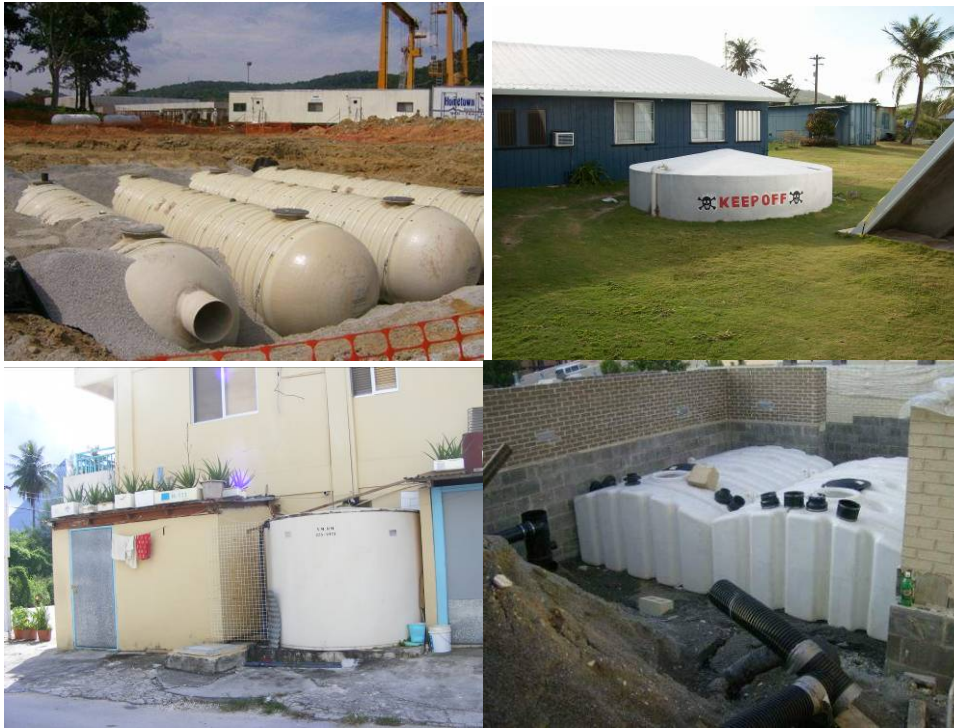
Figure S4.8. Various tank materials and configurations
