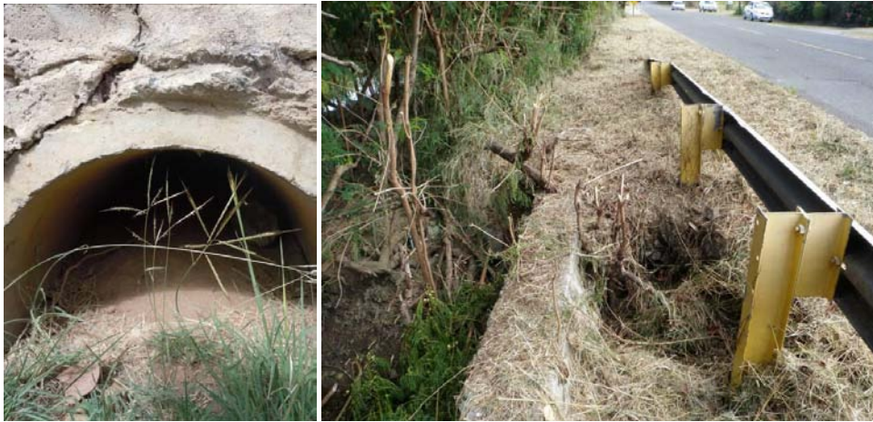
Figure 8. Blocked Culvert (Seven Flags) and Undermining of Culvert Headwall (Southgate East Gut)
