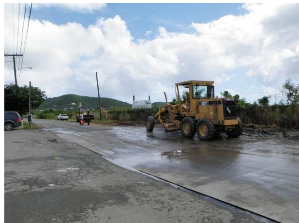
This area is a flooding nuisance and requires constant maintenance by DPW to clean out area where sediment settles and prevents drainage.
