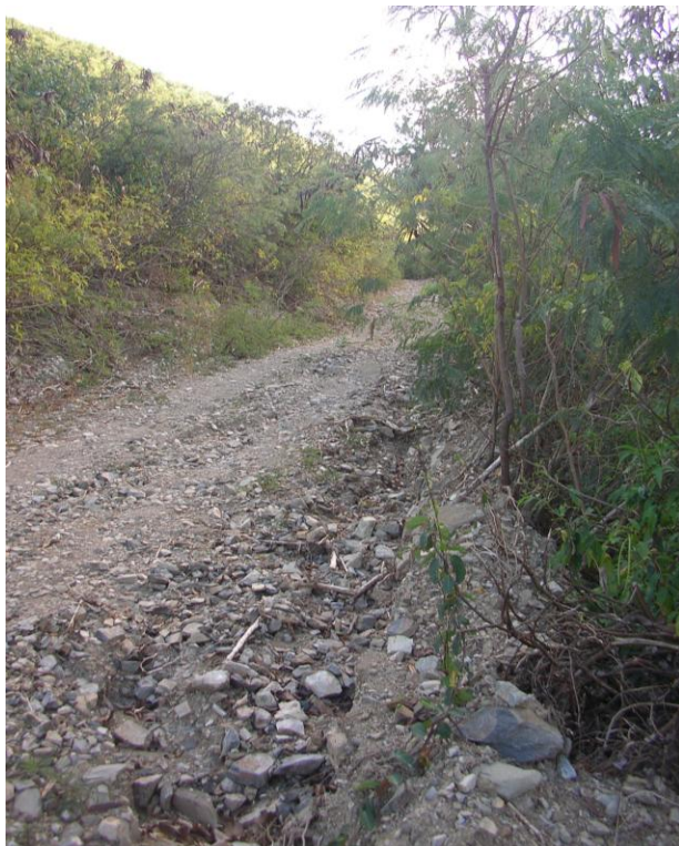
Erosion along ditch at upper portion of road.
