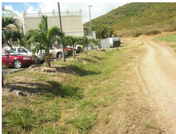
Existing swale along Ridge Rd. for proposed excavation and check dam installation. Install waterbars along road.
