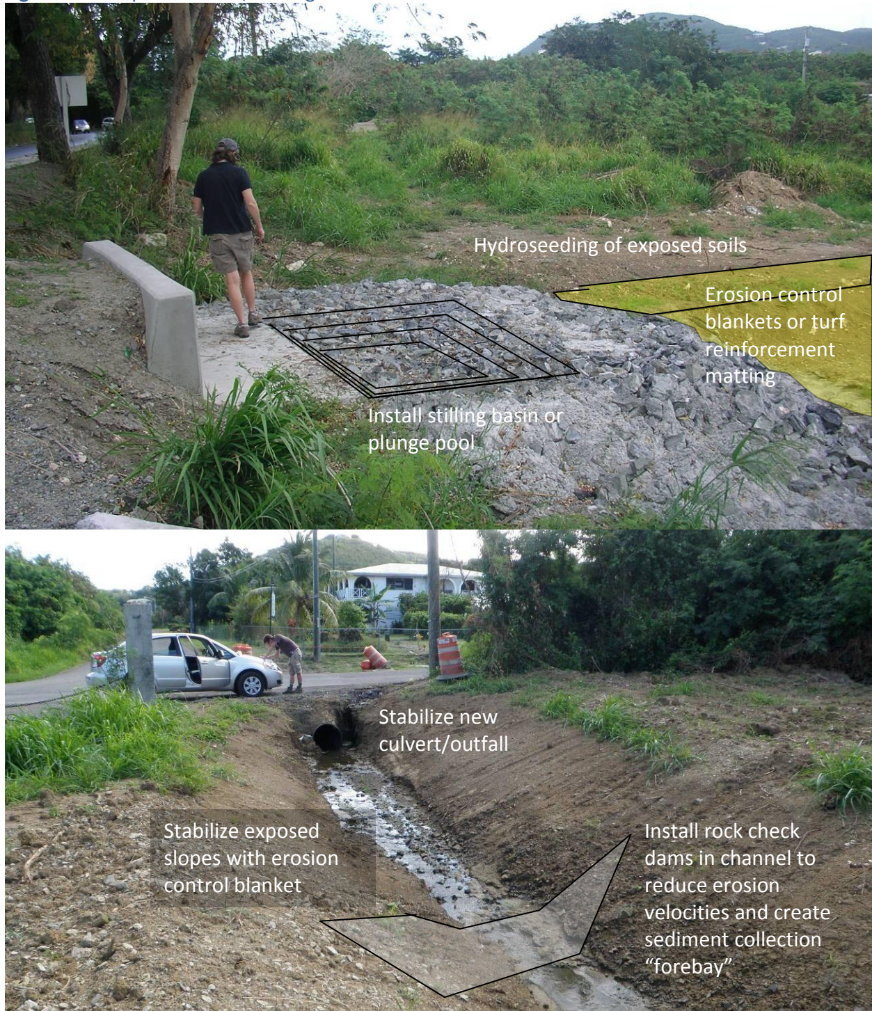
Figure 9. Example of Culvert/Drainage Outfalls in Need of Stabilization
