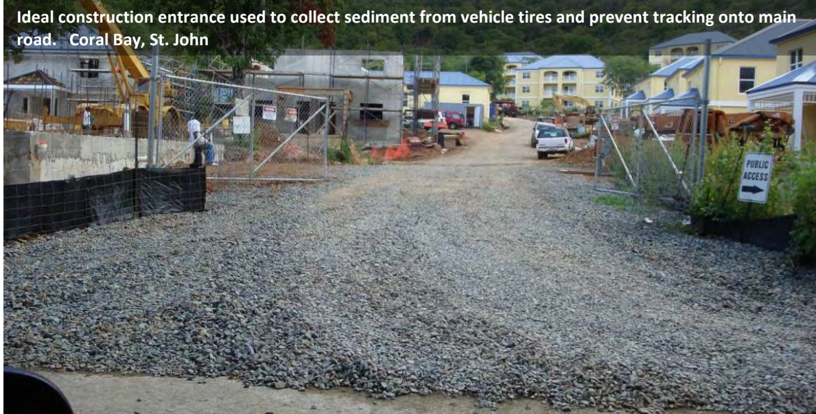
Geoweb installation on unpaved steep road in Coral Bay. This could potentially be used to stabilize the construction access road at site and/or installed on lower portion of road as a mechanism for holding gravel in place to reduce tracking of sediment off-site by construction vehicles.
