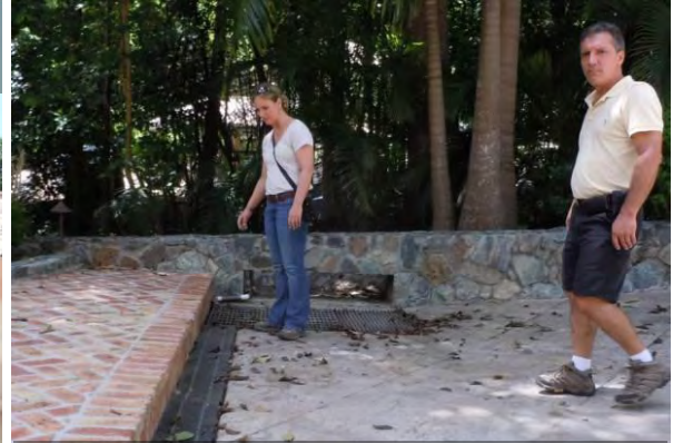
Stormwater runoff from driveway is collected via trench drain and stored in underground tanks for reuse in irrigation system.
