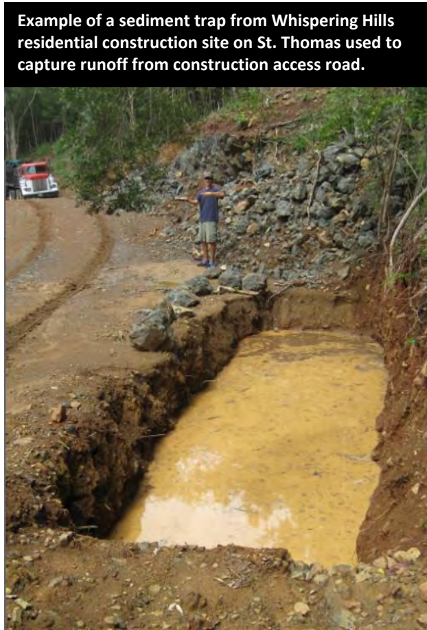
Figure 5A. Examples of sediment traps and dewatering basin.
