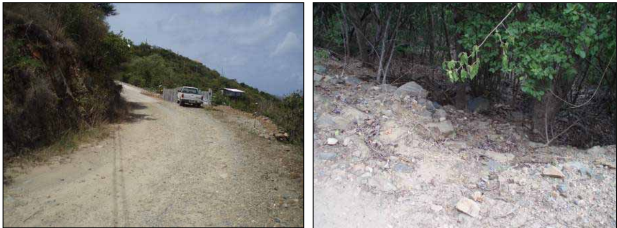
Figure 8. Hansen Bay Subdivision. Steep dirt road (left) and drainage through middle of subdivided property (right)
