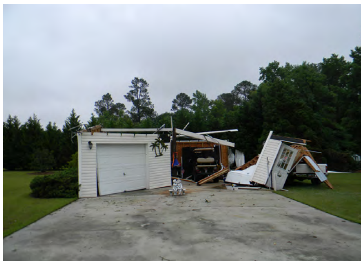
Downburst winds to 85 mph lifted and destroyed the detached roof two car garage at 800 pm EDT on 3/15/12. Debris was blown onto adjacent property as 3 2x4s pierced the mobile home outer wall. Considerable tree damage include a pecan orchard. Monetary damage was approximately $40,000. Photo taken by the Darlington County Emergency manager during a storm survey.
