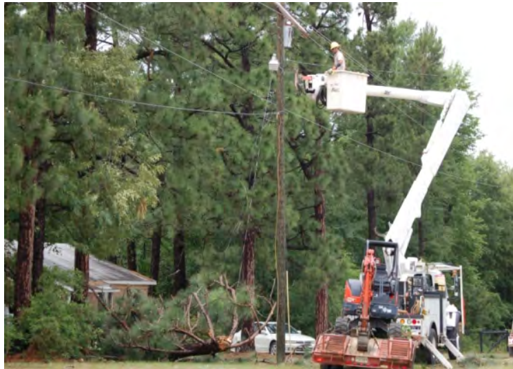
Linemen work to restore power after trees and powerlines came down. Photo by The Aiken Standard.
