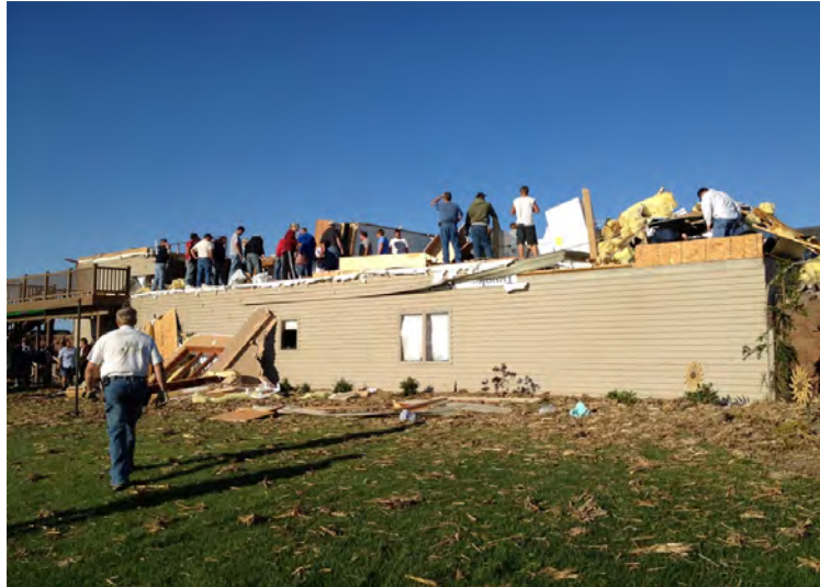
Damage to a rural home northwest of Cornlea, NE that was in the direct path of a tornado. Photo by Tim Hofbauer.
