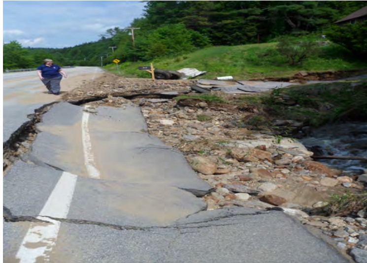
Flooding damage to Route 10 Northbound in Gilsum, north of Surry Road. Photo courtesy: Stephanie Dunten, NWS Storm Survey.
