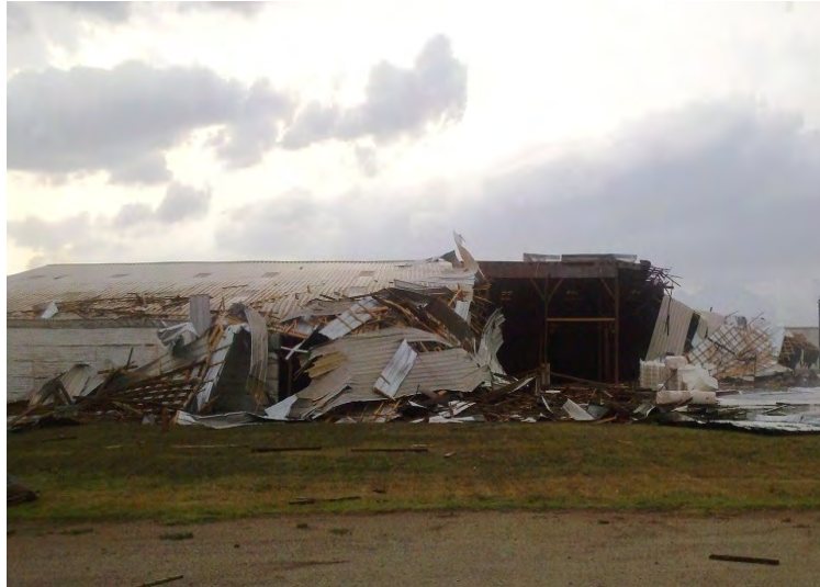
A portion of a warehouse on the north side of Paducah was heavily damaged by straight-line winds in the rear flank downdraft of an intense supercell. Photo courtesy of Kendall Stanaland.
