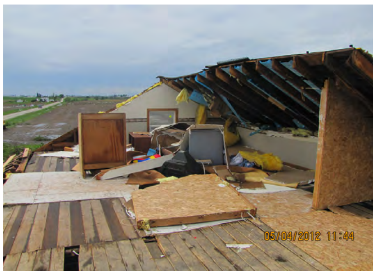
View from the upper floor of a home between Noble and Crawfordsville in Washington County of the damage done by a tornado.
