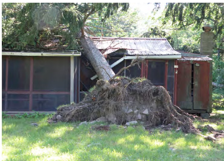
Large tree down on a summer cabin near Ingleby along Penns Creek in eastern Centre County. This was part of a larger damage swath (40-50 uprooted/snapped trees) associated with severe straight-line winds between 70 and 90 mph. Photo was taken as part of an official NWS Storm Survey.
