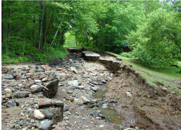
Back Road in Belvidere Vermont was washed out by Flash Flooding on May 29 2012. Photo by Paul Tamasi, used with permission.
