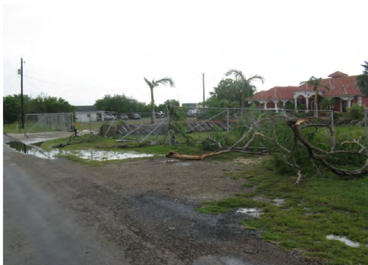
Damage to property and roof at a well built single family home in San Benito, TX from small tornado which contained estimated 80 mph winds. The large mesquite limbs were lifted from trees that could not be found on or near the property.
