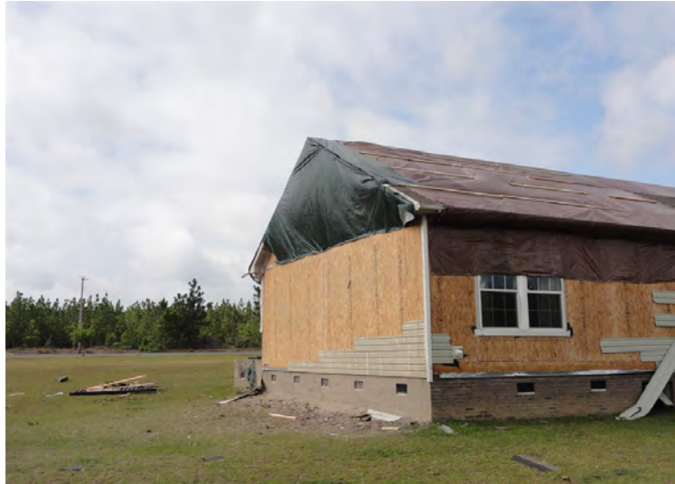
Rockingham EF-1 Tornado damage. May 16, 2012.
