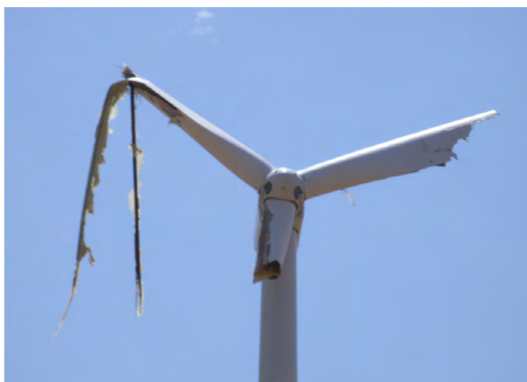
Damage to a turbine at the wind farm along the Harper and Kingman county line.
